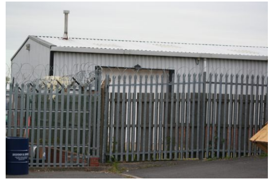
An example of an unsuitable boundary treatment
