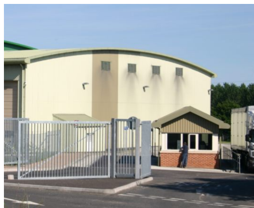
Poor elevational design, with vents staining the facade
