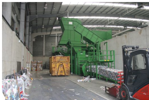
Bulking up facilities within a MRF
